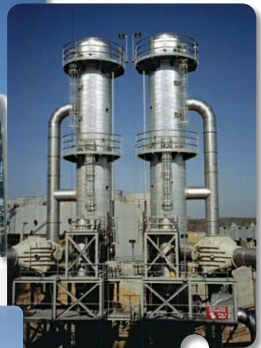
Cooling Tower Blowdown, Brine Concentrator
