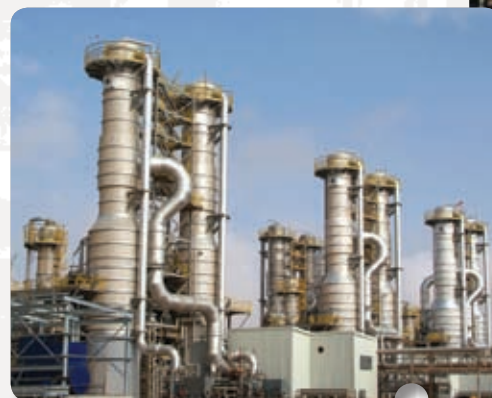
World's Largest Produced Water Evaporator System
