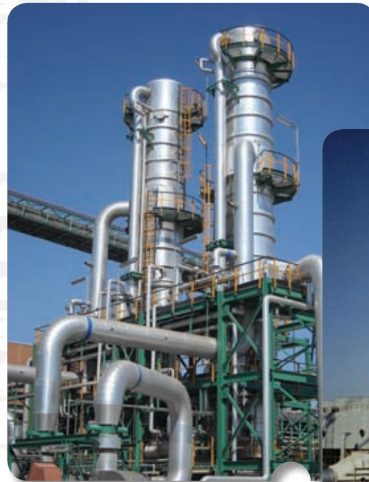
FGD Waste ZLD System
