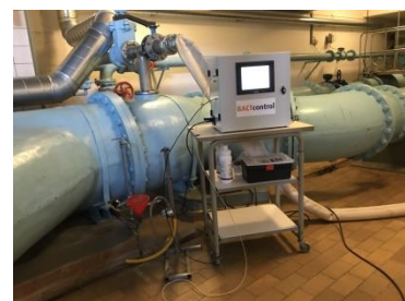
Fig.2 BACTcontrol in operation
